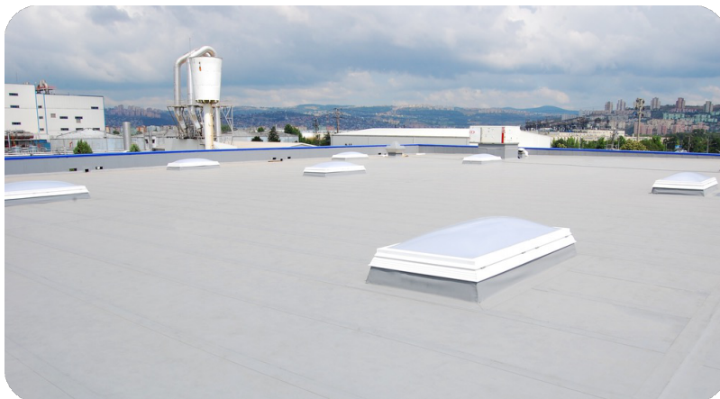
PIRBOARD under a single-ply membrane, large-span industrial roof
